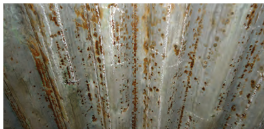
Waterwall after copper sulfate test
