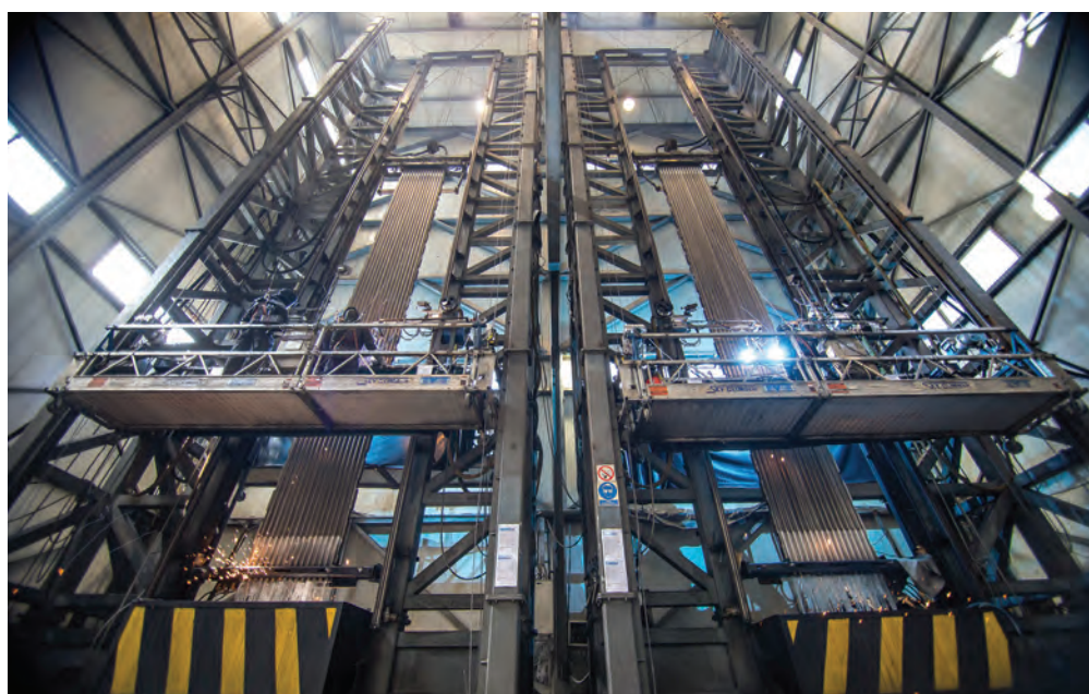
Boiler panel life extension
