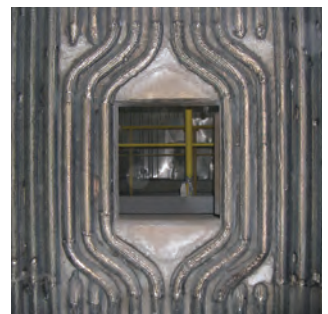
Spiral tubes with openings
