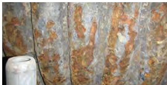
Fireside corrosion in a coal-fired boiler
